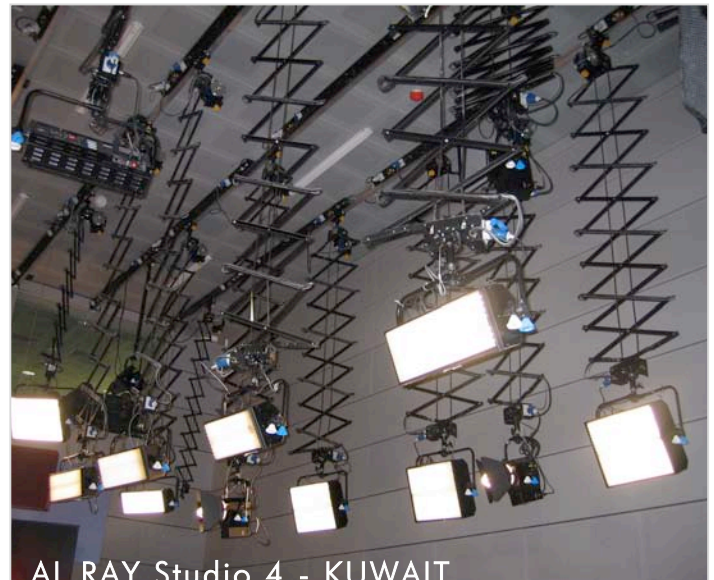
TYPICAL COLD LIGHTING DMX CONTROLLED (CST FRESNELS & FLUORESCENTS) INSTALLATION, USING THE "D" RAIL WITH INTEGRATED DMX AND MAINS ELECTRICAL DISTRIBUTION
